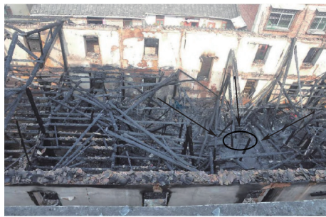
图 3 某建筑火灾中屋顶横梁倒塌情况 [9] (箭头指示横梁倒塌方向,圆圈标注位置为起火点) Fig. 3 A building fire causing collapse of roof crossbeam (arrows indicate fire origin area)
