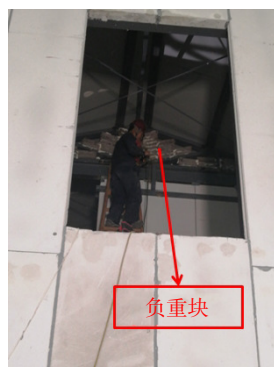
(e) 屋顶负重块 (e) Roof weight block
