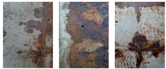
(a) 连接处裂缝 (b) 自由端裂缝 (c) 分布筋裂缝 (a) Cracks at junction (b) Cracks at free end (c) Cracks near distribution bars 图 5 试件表面锈胀裂缝 Fig. 5 Rust swelling cracks of specimens surface
