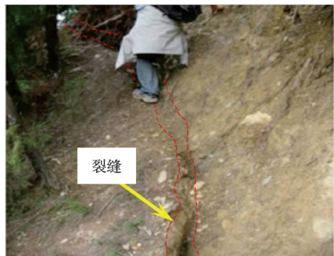
(b) 青川县红光乡三元坝边坡裂缝 (b) The crack of Sanyuanba slope in Hongguang town Qingchuan county
