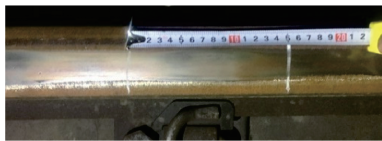
(b) 钢轨波磨调研现场 (b) Field investigation of rail corrugation
