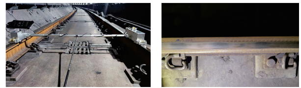
(a) 钢轨波磨仪 (b) 钢轨波磨 (a) Rail corrugation measuring instrument (b) Rail corrugation
