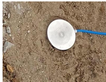
图 3 现场埋设土压力盒照片 Fig.3 Photograph of field embedding of soil pressure cell
