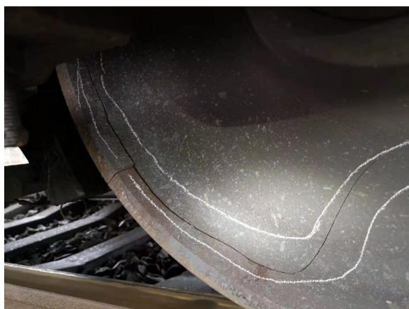
a circumferential crack of 468 mm
