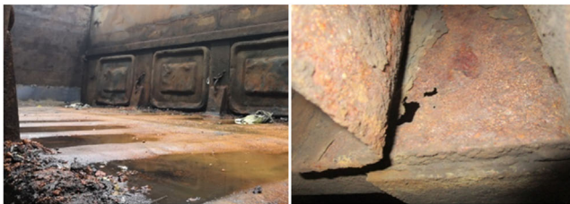
Figure 1. Corrosion of freight. Source(s): Authors' own work
