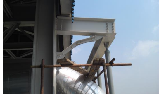
图 1 管道下沉及刚性吊架三角架斜撑弯曲失效 Fig.1 Pipe sinking and rigid hanger tripod sway bending
