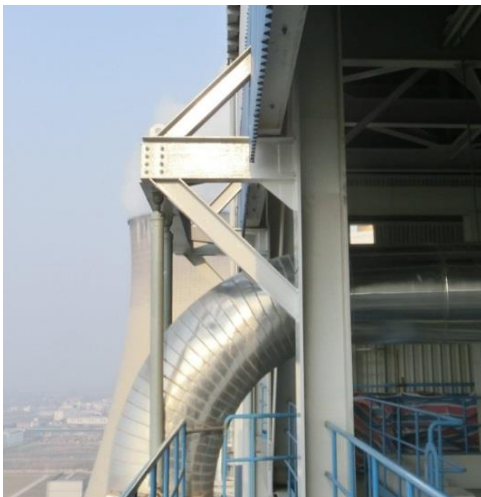
图 7 改进后刚性吊架三角架斜撑 Fig.7 The improved rigid hanger triangle sway
