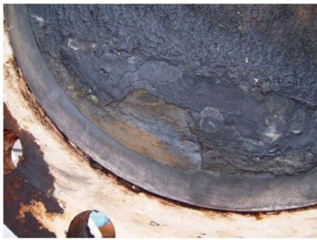
图 1 海底金属管道 CO 2 腐蚀 Fig.1 CO 2 corrosion of submarine metal pipeline
