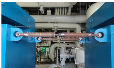
图 6 径向支撑现场安装方式 Fig.6 Field installation drawing of radial support
