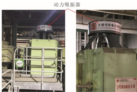
图 9 凝泵电机顶部动力吸振器布置现场 Fig.9 Layout of the dynamic vibration absorber upon the condensate pump motor
