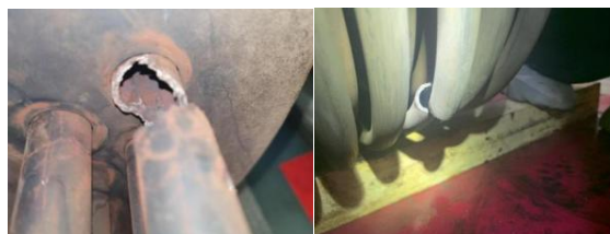
图2 某电厂尿素水解器盘管应力腐蚀破裂( \text{Cl}^- 导致) Fig.2 The stress corrosion rupture of urea hydrolyzer coil in a power plant (caused by \text{Cl}^- )
