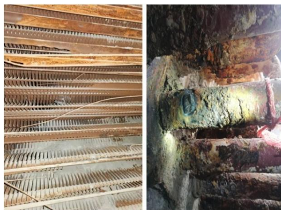
图 4 烟气冷却器磨损泄漏及弯头腐蚀泄漏 Fig.4 The wear and tear leakage and elbow corrosion leakage of flue gas coolers
