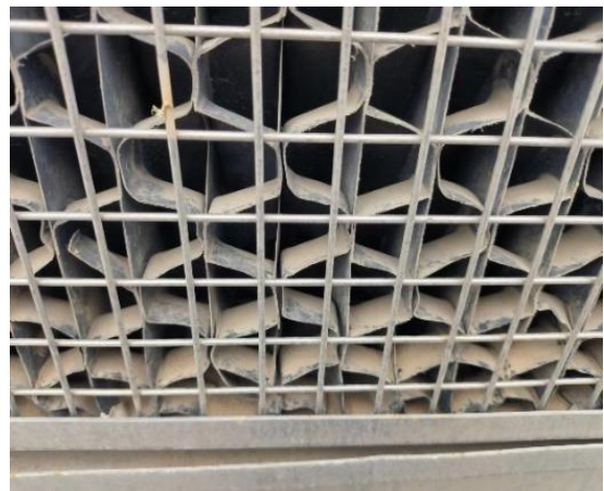
图10 蒸发冷却器防尘网风沙侵入情况 Fig.10 Dust intrusion of evaporative cooler air filter
