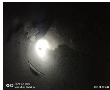
图14 过热器 TP91 管段铁氧化物沉积和剥离管样 Fig.14 Iron oxide deposition and stripping sample of TP91 superheater
