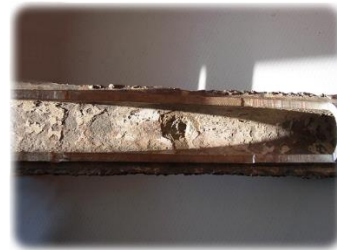
图 4 水冷壁钙镁垢和腐蚀坑 Fig.4 Water wall scale and corrosion pit
