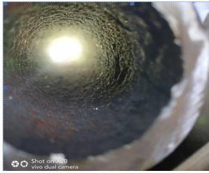
图9 水冷壁管段铁氧化物沉积 (237 g/m 2 管样) Fig.9 Iron oxide deposition in water wall pipe section (237 g/m 2 pipe sample)
