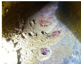
图 22 某 12Cr1MoV 再热器 U 型管排底部穿孔泄漏宏观图 Fig.22 Macro view of perforation leakage at the bottom of U-shaped tube bank of 12Cr1MoV reheater
