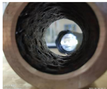
图 8 省煤器进口管段铁氧化物沉积量 ( 460 \text{ g/m}^2 管样) Fig.8 Iron oxide deposition in the inlet pipe section of economizer ( 460 \text{ g/m}^2 pipe sample)
