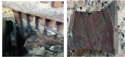
图 24 工字钢与风箱焊接部位炉管爆管 Fig.24 Furnace tube explosion at the welding position of I-beam and bellows
