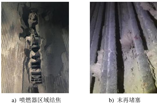
图 2 125 MW 机组锅炉燃烧器区域和末再积灰堵塞情况 Fig.2 Ash blocking of burner zone and final reheater of 125 MW boiler
