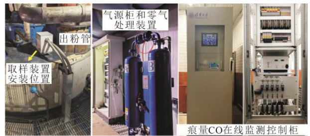
图 8 350 MW 磨煤机 CO 在线监测现场应用示范 Fig.8 Field application demonstration of 350 MW Coal Mill CO online monitoring
