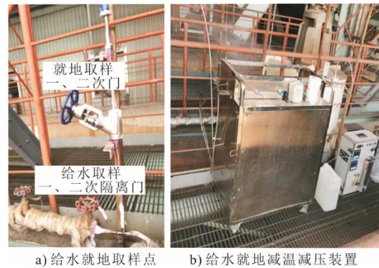
图 1 给水就地取样点及就地减温减压装置 Fig.1 The local sampling point of feed water and local temperature and pressure reducing device
