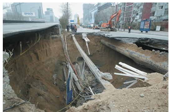
图1 北京市呼家楼小区附近道路塌陷事故 Fig. 1 Road collapse near Hujialou neighborhood, Beijing, China
