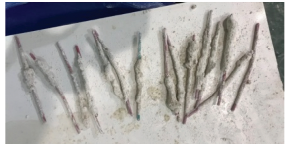
图 6 锚杆受载后破坏图 Fig. 6 The failure of bolt anchorage
