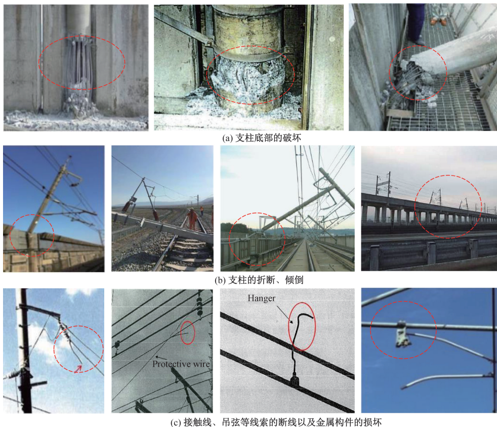
图 3 接触网破坏情况 [8,45-50] Fig. 3 Condition of the OCS damage [8,45-50]
