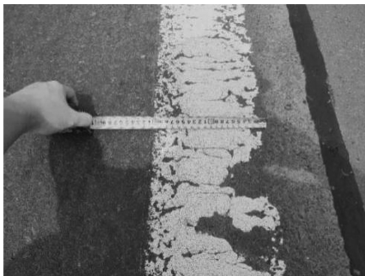
(c) 涂料脱落
