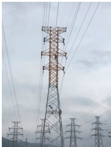
图1 浙江丽水110 kV遂溪1094线路同杆架设的FRP杆塔 Fig. 1 FRP Transmission Tower on 110 kV Suixi 1094 Line of Zhejiang Lishui
