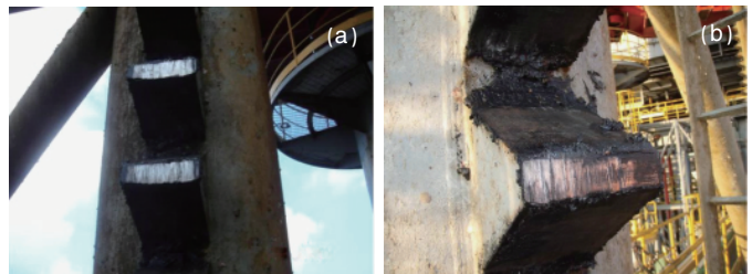
图 3 齿条磨损 Fig. 3 Wear and damage in racks
