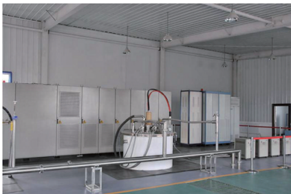
图 9 超导变电站中的 1 MJ/0.5 MV·A SMES Fig. 9 1 MJ/0.5 MV·A SMES installed at the superconducting power substation
