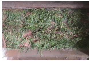
图4 三维网草皮被冲刷 Fig. 4 Three dimensional mesh cushion grass
