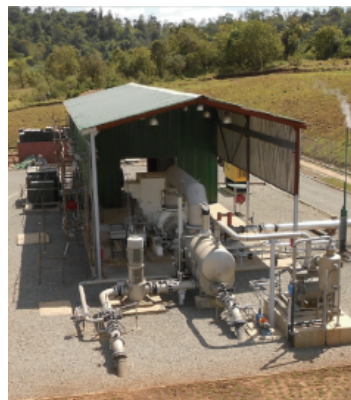
图 10 井口发电设备(发电机、冷凝器、冷水泵等) Fig. 10 Power generator, condenser and main cooling water pump
