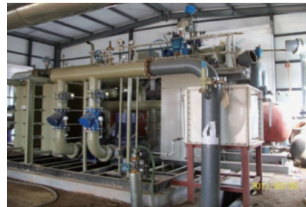
图 11 华北油田地热发电双工质螺杆膨胀机 Fig. 11 Binary screw expander used for geothermal power generation in Huabei Oilfield
