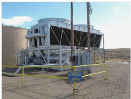
图 10 250kW 有机朗肯循环 (ORC) 低温地热发电系统 Fig. 10 Geothermal power generation system of 250kW organic Rankine cycle using low temperature geothermal resource
