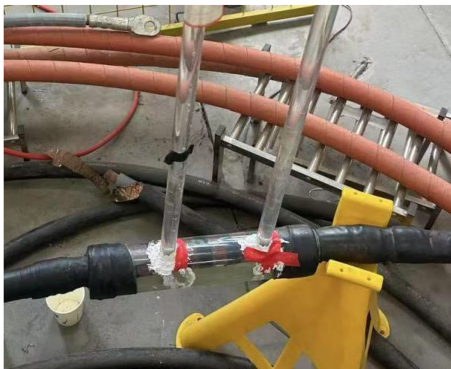
图6 电缆进水受潮试样 Fig.6 Cable samples with water ingress and moisture
