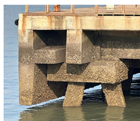
(a) Oysters densely coating a pier at Tianjin Port
