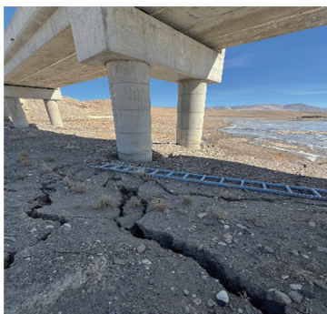
(c) 贯穿桥梁的地表裂缝
