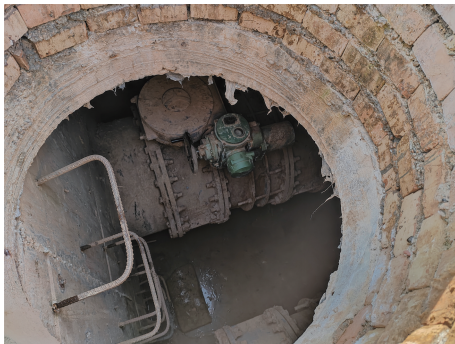
图 5 阀门井中管道连接处轻微渗漏 Fig. 5 Minor leakage at pipe connections in valve shafts
