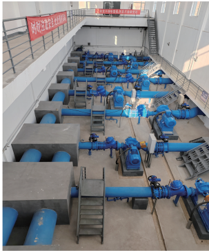
图 2 泵房内 8 部出水阀电泵 Fig. 2 Eight outlet valve electric pumps in the pump house
