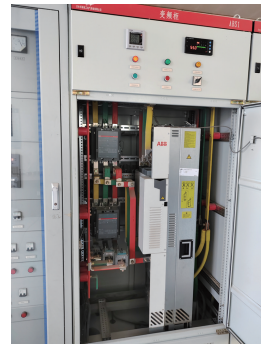
图 6 倾覆的变频柜在震后 30 min 复位 Fig. 6 Overturned inverter cabinet rest 30 minutes after the earthquake
