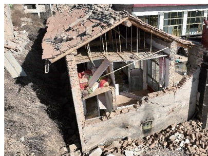
(c) 侧面局部倒塌
