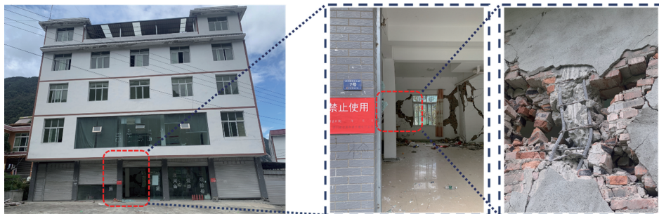
图 7 得妥镇南头村某 5 层建筑 Fig. 7 A five stary building in Nantou Village, Detuo Town
