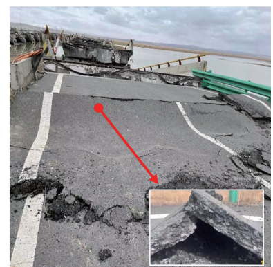
(c) 边坡路面挤压隆起
