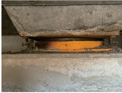
图 7 北侧支座处连接锚栓折断 Fig. 7 Broken of the anchor bolt of the north support
