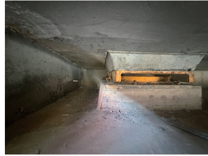
图 8 北侧单向支座连接锚栓被挤压倾斜 Fig. 8 Extruded and tilted of the anchor bolt of the one-way support on the north side
