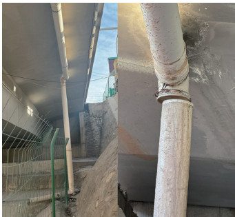
图 9 排水管拉脱 Fig. 9 Pulled of the drainpipes
