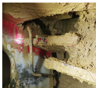
图 13 刀盘上缠绕钢筋 Figure 13 Wrapped steel bars of cutter-head
