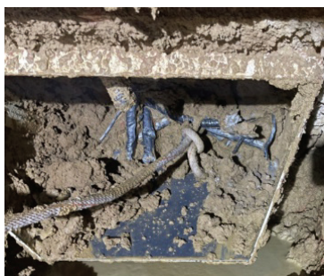
图 12 螺旋机出渣口钢筋清理 Figure 12 Reinforcement cleaning of screw slag outlet
