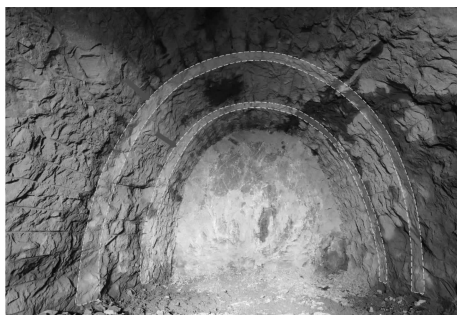
图 8 错台过宽导致超挖较大 Fig. 8 The platform is too wide causing overcut
