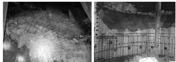
(a) 上分层施工情况 (a) Construction situation of upper layer (b) 中分层(下分层)施工情况 (b) Construction situation of middle layer (lower layer)
