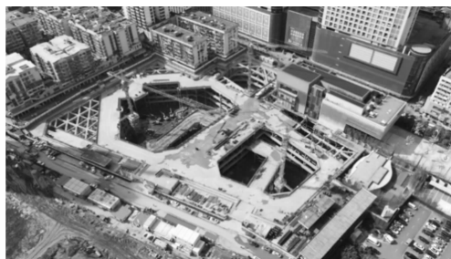
图1 深基坑支撑梁体系与周边环境图 Fig. 1 The deep foundation pit supporting beam system and its surrounding environment
