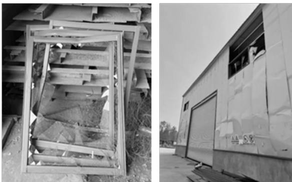
(a) 脱落的窗框 (b) 彩钢房外壁 (a) Dislodged window frames (b) Outer wall of the color steel room
