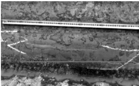
(a) 渣沟裂纹
